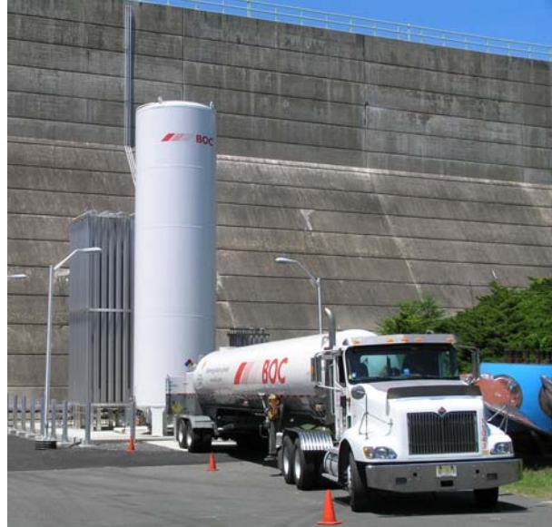
Figure 4: Shepaug Oxygen Supply Facility
