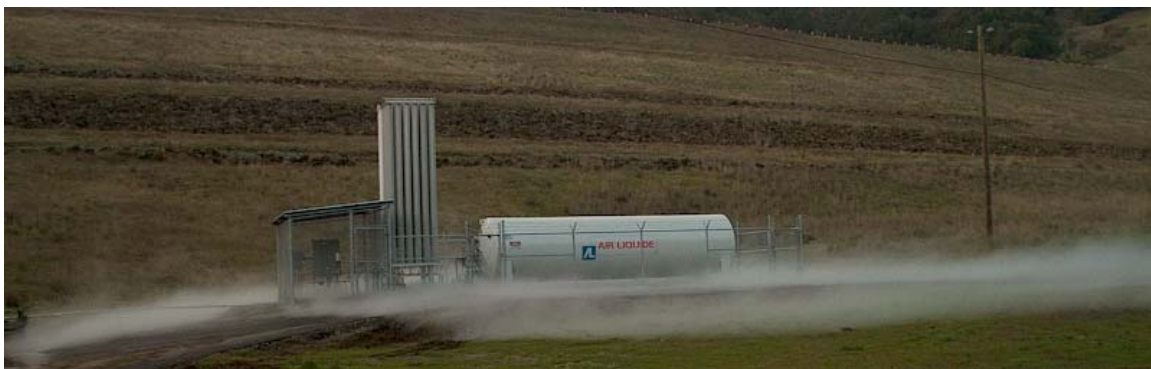
USL Oxygen Supply Facility
